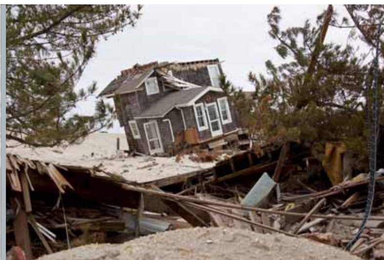
A house lifted from its foundations on the beach on 13 January 2013 in Mantoloking, New Jersey. Clean-up continued 75 days after Hurricane Sandy struck in October 2012.
